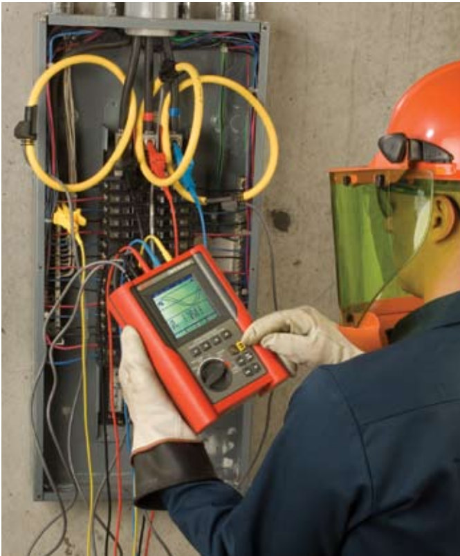
Check for the presence and level of harmonics by measuring current on the feeder at neutral, which will typically be in the 80 percent to 130 percent range.
